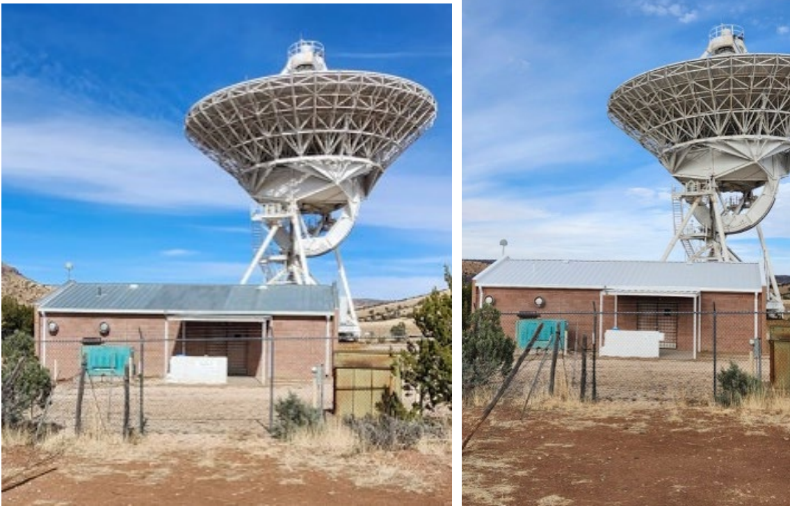
Image 1-2: (L) Fort Davis site, before roof replacement. (R) Fort Davis, after roof replacement.
